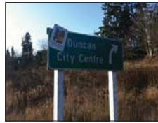
A-02 M.T.I Directional Sign 1. Currently directs travellers to the Sherman Rd./Canada Ave roundabout. 2. Recommend that MTI removes this sign.
