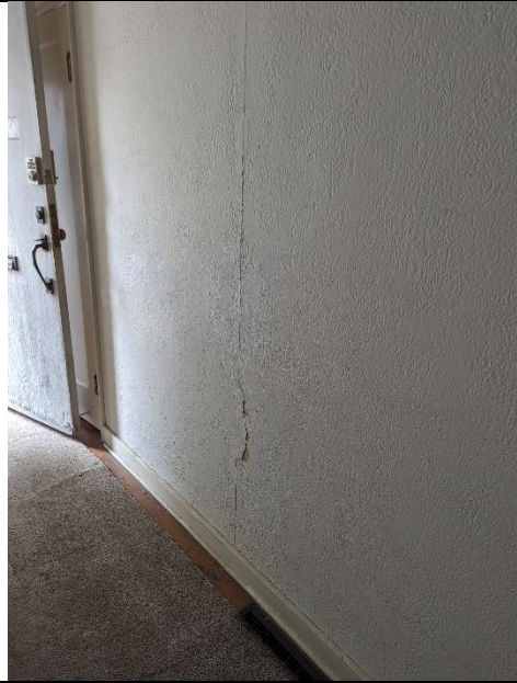
Sample: 50288 – 2 Location: Living Room – Wall Description: Drywall Joint Compound/Textured Coating Asbestos: Chrysotile 1%
