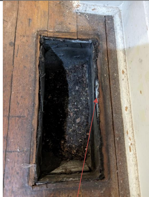
Sample: n/a Location: Dining Room – Heating Vent Description: Typical View of Asbestos Containing Fibreboard Asbestos: Typically, 60% Chrysotile
