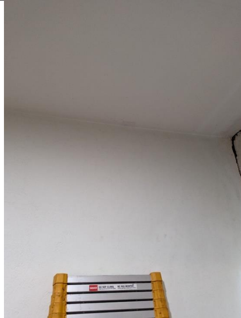
Sample: 50288 – 4 Location: Dining Room – Ceiling Description: Drywall Joint Compound/Textured Coating Asbestos: Chrysotile 1%
