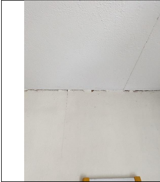
Sample: 50288 – 1 Location: Living Room – Ceiling Description: Drywall Joint Compound/Textured Coating Asbestos: Chrysotile 1%
