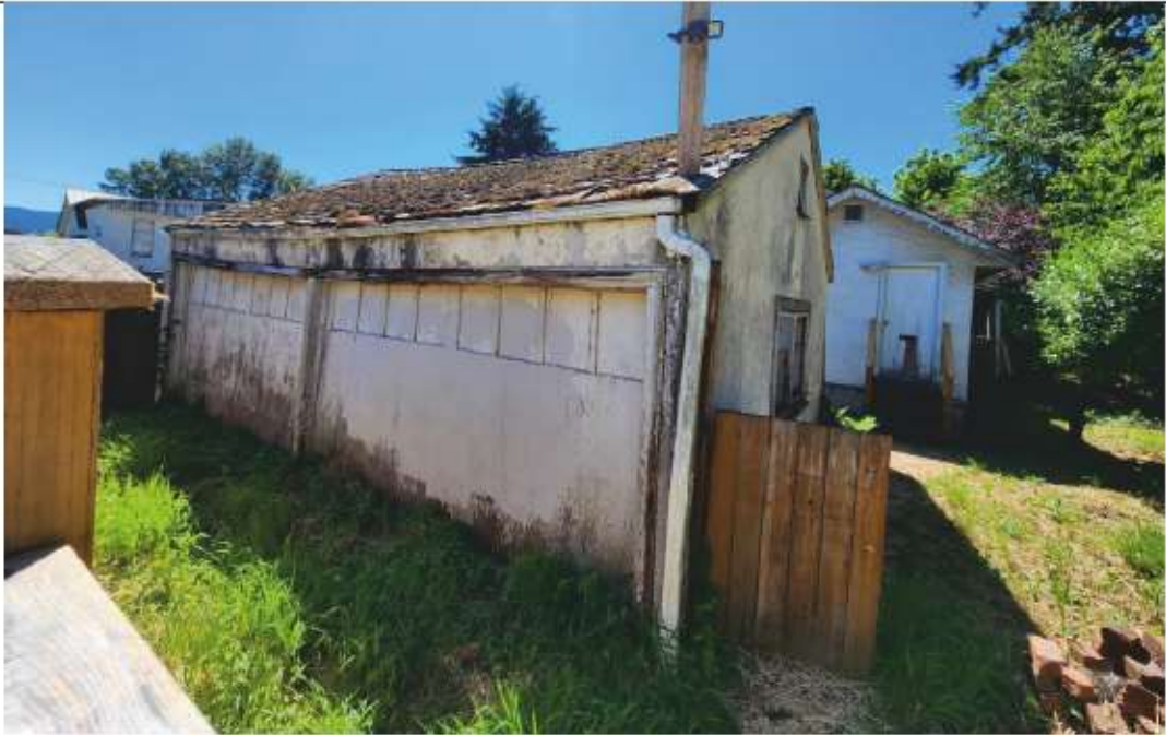
Photograph 5 Photo showing the two-car garage located at the rear of the property. Photo taken from the north property boundary looking south.
