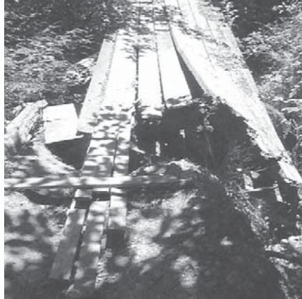
The bridge near Cassino Road is in poor condition.
