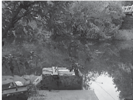
The existing foundations on the south side of the Chemainus River bridge could be used to build a separate TCT crossing.
