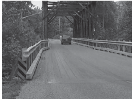
The existing bridge deck is dangerous because of the rough surface and narrow width.
